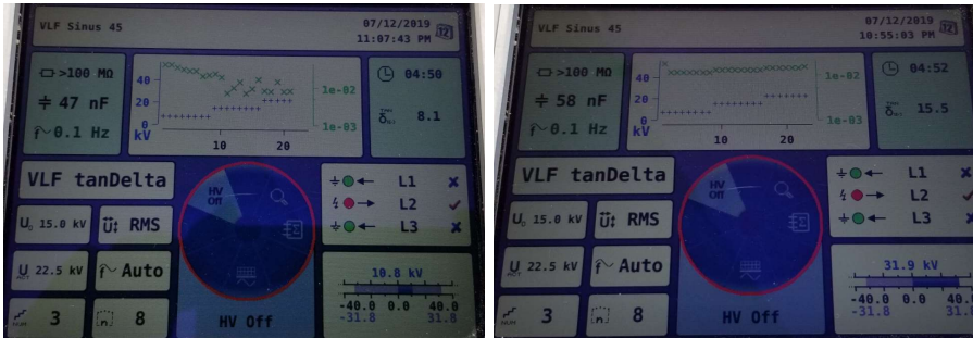
Figure 13: The screen capture on the left demonstrates the impact of testing in high-humidity conditions. The results do not align with expected results. The screen capture on the right is the same cable after multiple tests. Results stabilized after a dry out period along with other physical mitigation measures. Compared to results in Figure 12, these results are aberrant due to high humidity.
