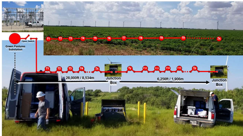
Figure 18: Example of long-continuous runs of cable with limited sectionalizing capabilities for both CFL and CTD activities. 28,000ft segment between substation and Junction Box create a challenge for cable test activities. Design recommendation for similar installations would be to recommend that a junction-box is installed within the 28,000ft run of cable to aid in future maintenance efforts.
